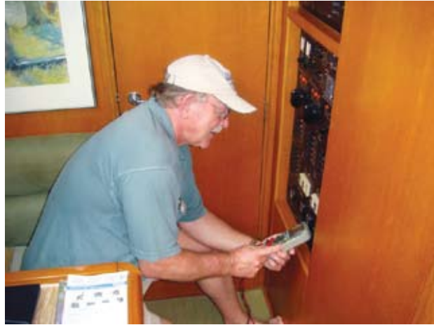
The insurance surveyor checking through Lulu's electrical system
