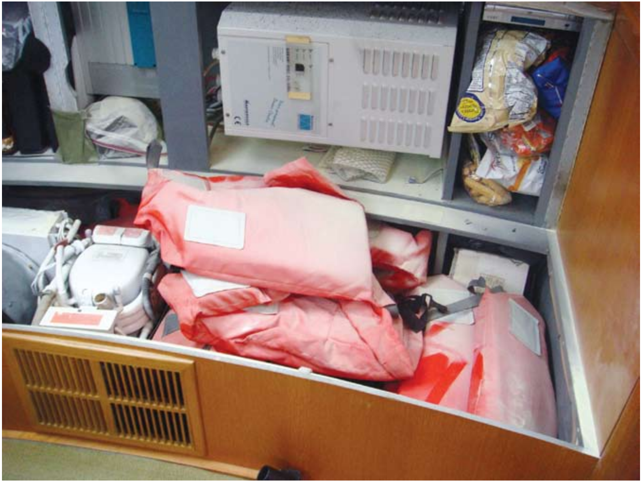
The fried inverter with the fire extinguisher mess, above. Lulu at the "other" marina, opposite
